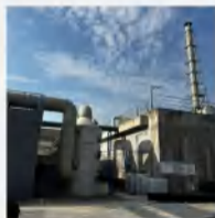
■ Sludge Drying and Deodorization facilities
